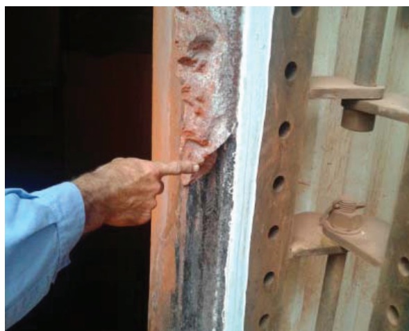
Figure 9. Crust formed on the inside wall of the tank.
