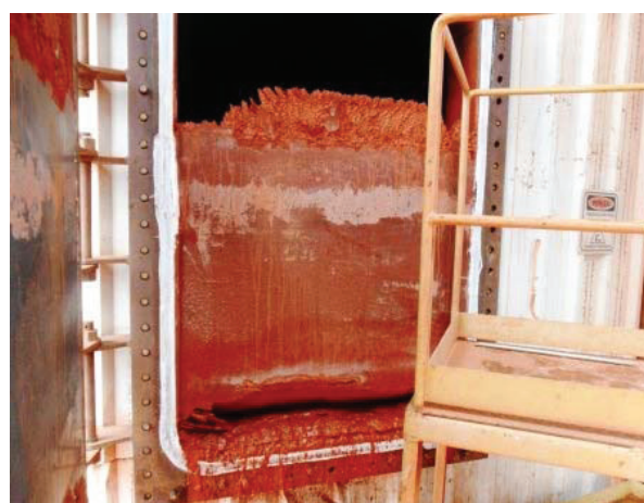
Figure 7. Crust formed on the inner wall of the tank
